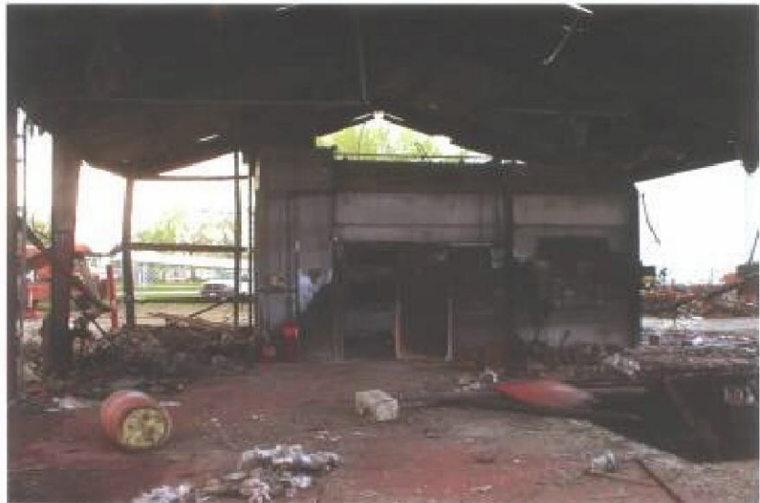
The fire damage at Kelly Ryan Manufacturing destroyed their paint booth building and caused severe smoke and heat damage to adjoining structures.
