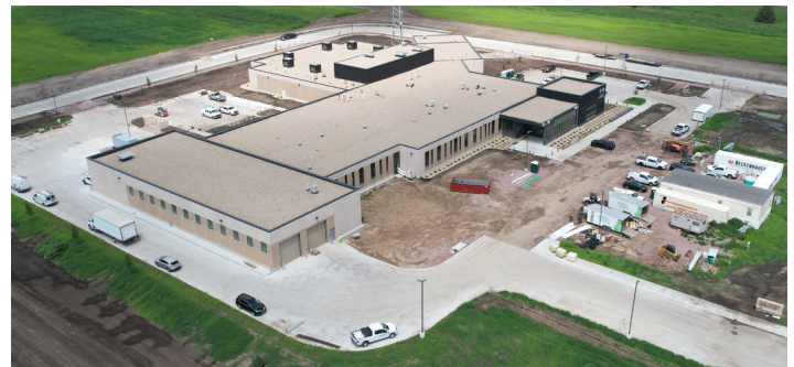
The 62,500SF facility is nearing the finish line, soon to home the Vermillion Police Department and Clay County Sheriff's Department.
