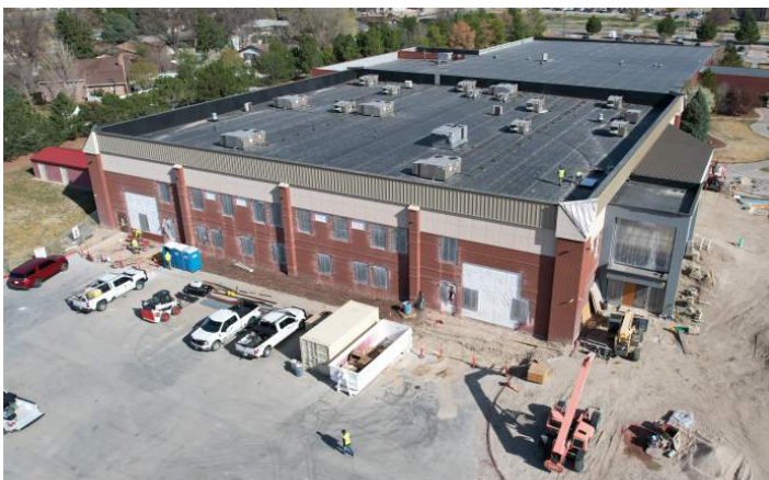
This project is 33,000 SF of renovation with a 1,160SF addition which will provide WNCC with a modern facility for their students.
